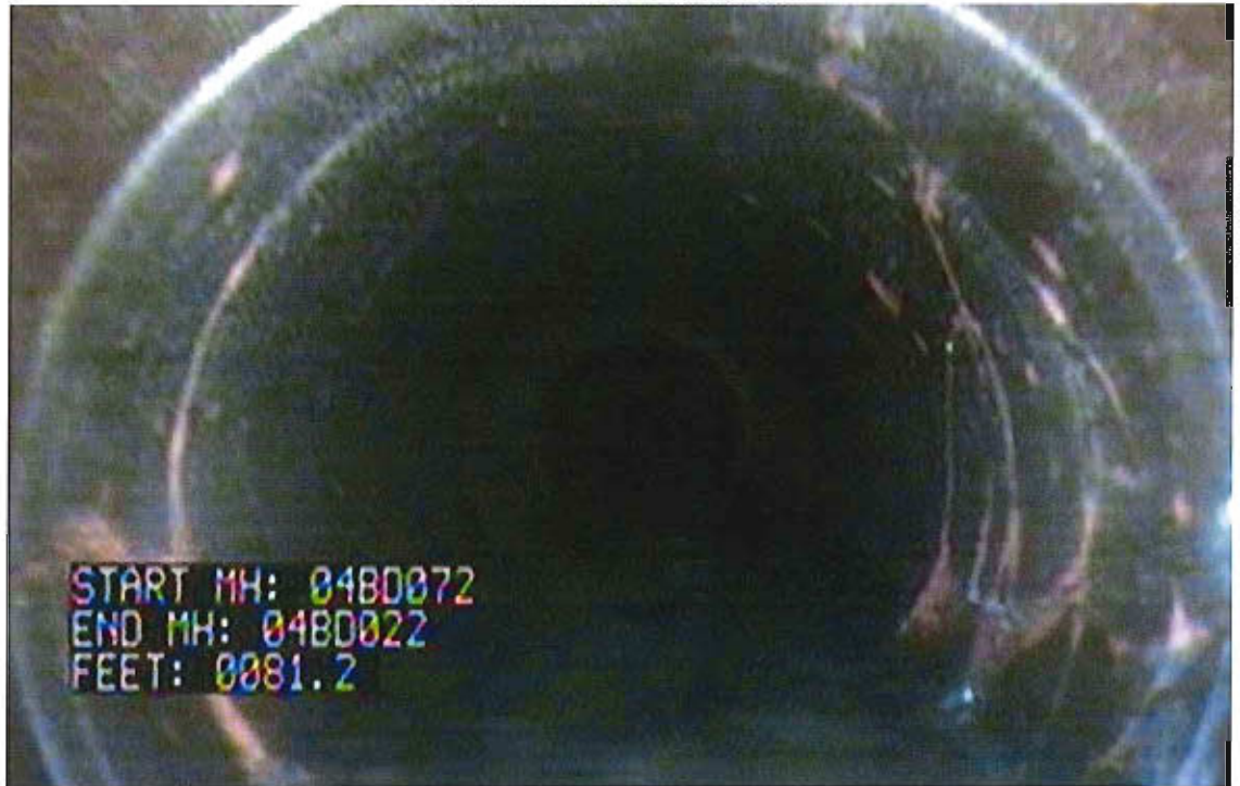
Cracks and fractures forming at the sides
