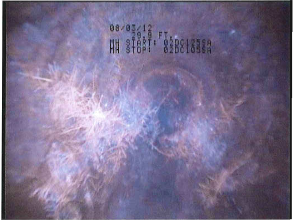
Roots at pipe joints
