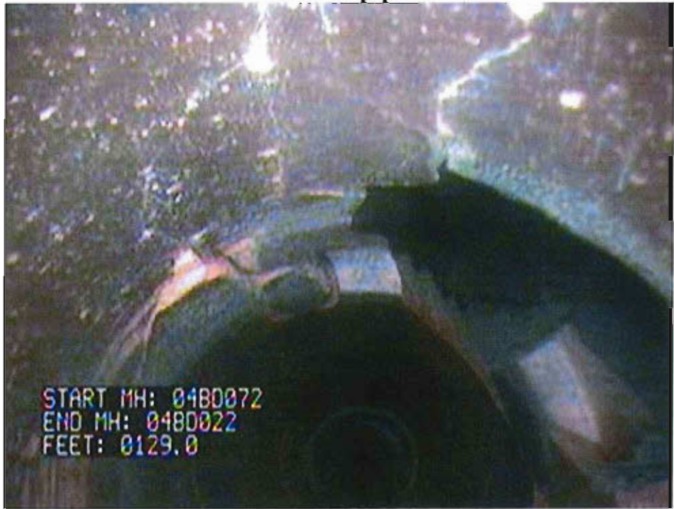
Hole at top right of 8" clay pipe
