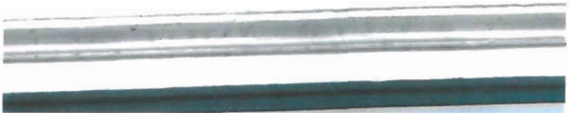
Stained glass to be repaired.
