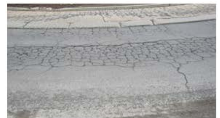
Pavement inlay needed
