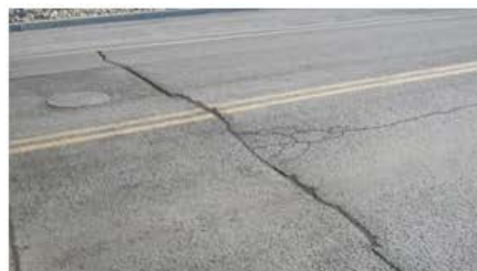
Pavement overlay needed
