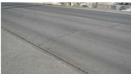
Crack seal and chip seal needed
